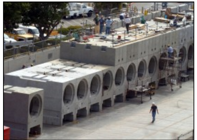
San Onofre dry cask storage system
